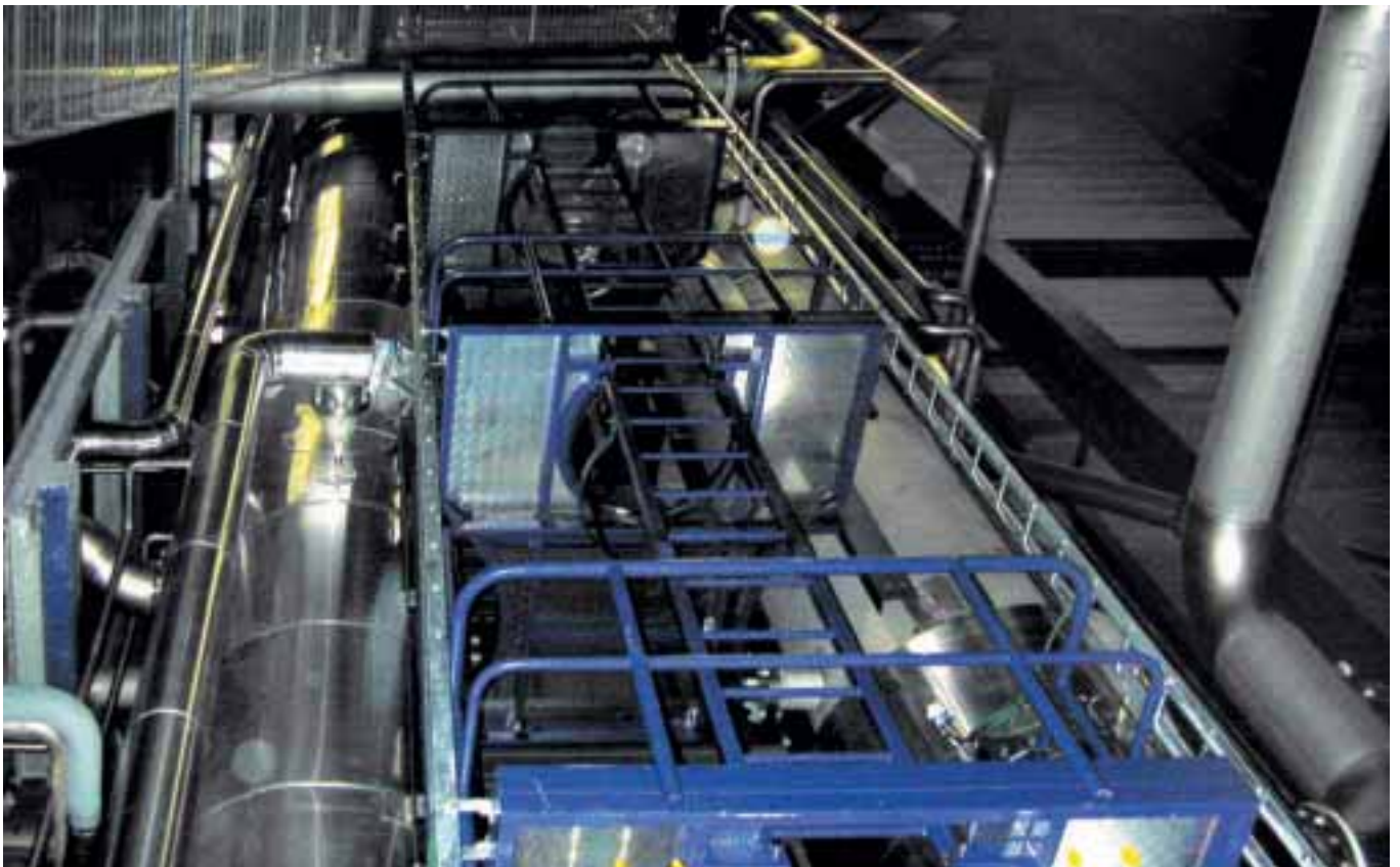
Pilot CO 2 capture facility. European Castor project (Dong – Esbjerg site, Denmark).
