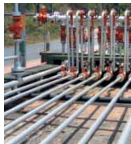
Pilot CO 2 injection facility.
