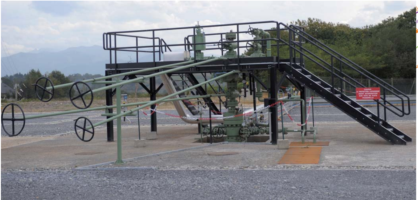
Well-head used for the CO 2 injection: the Total pilot unit is being used to test an integrated project for the geological capture and storage of CO 2 in the Lacq basin.
